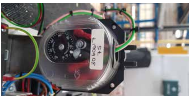
Figure 23b : Kromshrode air pressure switch
