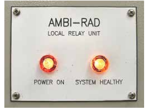
Figure 3. Inverter panel (behind hinged cover)
